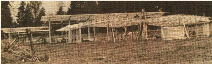
School Construction Underway: Although they are working against adverse weather conditions which have transformed the site into a sea of mud, workmen still hope to have the Ballinger Elementary School completed in time for occupancy next September. (44)
